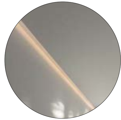
Gyp Ceiling With Cove Light
